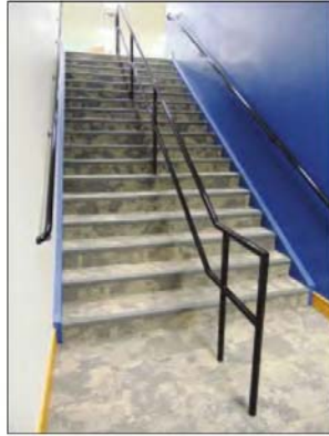
A center handrail was installed along the main staircase photos by Jeff Lysiak
